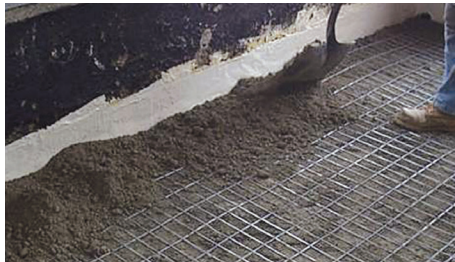
Figure 7.11 — Example of a non-bonded, wire reinforced mortar bed. Wire mesh is placed in the middle of the mortar bed and lapped together to ensure continuity. Notice that the mortar below the wire mesh has been compacted, thus ensuring that the entire mortar bed is compacted properly.
