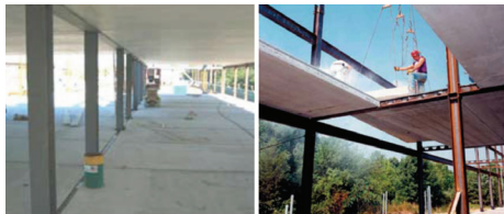
Figure 2.25 – Pre cast concrete planks. Planks rest and are supported by a flange attached to the steel girders. The planks are hoisted into place by a crane and mortared to the beams and to each other. Photo courtesy of Girder Slab Technologies LLC.
