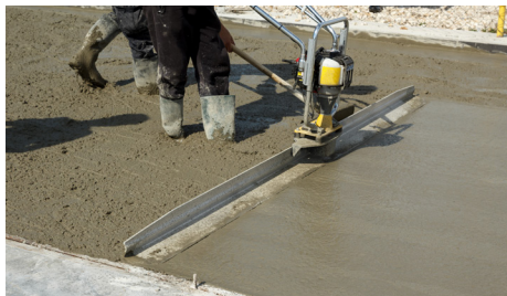
Figure 8.23 – Mortar is screeded with a vibrating screed to the desired height and pitched to falls and drains as required.
