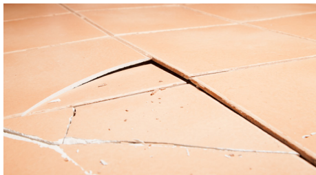
Figure 2.4 — Result of stresses induced by concrete shrinkage and lack of movement joint control. As the concrete shrinks, expansion joints are required to relieve the stress. When expansion joints are omitted or are not sufficient, “tenting” of the tiles can occur, creating bond failure and cracking.
