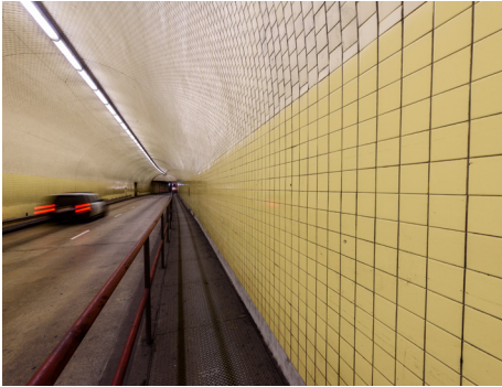
Figure 5.4 – Robert C. Levy Tunnel, better known as the Broadway Tunnel in San Francisco, California.
