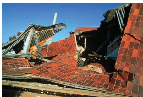
Figure 7.2 — High adhesive shear and tensile strength to resist seismic movement. Photograph of the Bullocks building after the Northridge, CA earthquake in 1994. Tiles remain adhered after severe shear stress from seismic activity and structural failure.
