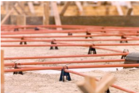
Figure 2.23 – Post tensioned concrete cables. Notice the orange tensioning cables that will run throughout the concrete slab. Photo Courtesy of SunCoast Post Tensioning Company.
