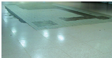
Figure 8.27 – Restoration of the St. George Ferry Terminal, New York, NY included the installation of new tile over existing cement based terrazzo and tiled floors.
