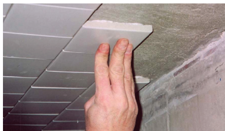
Figure 8.26 – Restoration of the Route 9 Tunnel, New York, NY. Installation of new ceramic tile over existing concrete ceiling using LATAPOXY® 310 Stone Adhesive in the epoxy spot bond method. Installation by Navillus Contracting Inc., Long Island City, NY.
