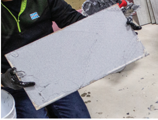
Figure 7.9 – Ceramic tile removed during the installation to verify proper coverage is being attained. Notice the lower right hand corner of the tile is locking coverage. This could well lead to a cracked tile.
