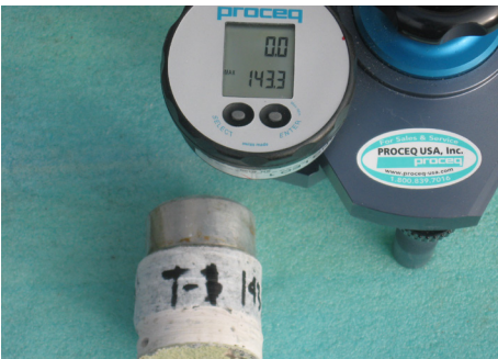
Figure 9.8 – View of cored stone and adhesive section. In this instance, failure occurred at the waterproofing membrane to substrate interface at approximately ~143 psi (1 MPa) (very good results).
