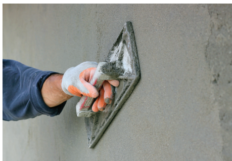
Figure 7.14 – Tile mechanic applying latex fortified cement based scratch coat to a block wall with a hawk and trowel.
