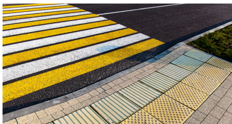
Figure 5.10—ADA Compliant Detectable Warning Tile Installed next to a roadside pedestrian crossing.
