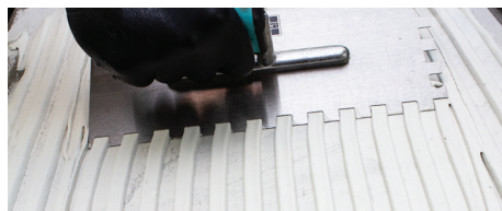
Figure 7.5 – Trowel applied medium bed mortar with a 3/4" (19 mm) square notch trowel used for large format tiles or stones. Trowel medium bed mortar in one direction holding trowel at a 45 degree angle. Notice the full ribbons of mortar that are left behind.
