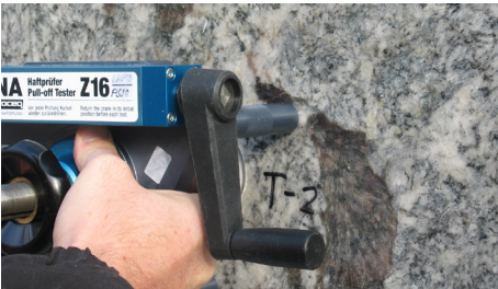
Figure 9.7 – Portable tensile pull testing equipment is attached to the metal disc. Test equipment exerts a "pulling" force on the disc and cored stone section (to the point of failure) to measure its tensile bond strength.
