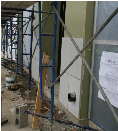
Figure 8.2 — Exterior façade work in temporarily heated, tented area in the middle of winter. LATICRETE Headquarters building, Bethany, CT.
