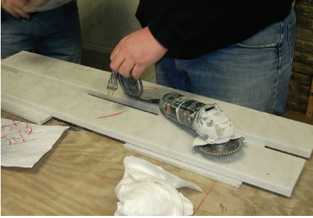
Figure 7.16 – Stone is prepared for installation by the epoxy spot bond method. Stone back is roughened at the adhesive connection points then washed and allowed to dry.
