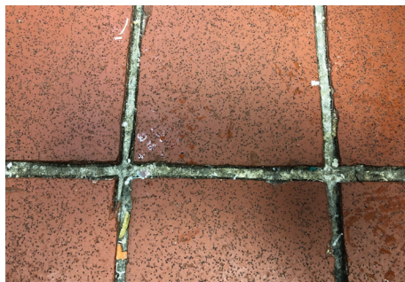
Figure 7.20 — Effects of inappropriate grout used on a demanding application. Notice not only the erosion of the grout joints, but also the adhesive mortar under the tile. In many floor applications, the use of an epoxy based adhesive and grout are required in order to ensure long-term performance.
