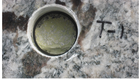
Figure 9.9 – View of cored stone remaining on vertical wall surface.
