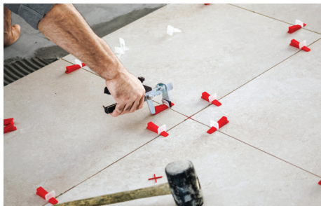
Figure 7.4 – Tiler placing ceramic tile in position over adhesive with tile levelling system.
