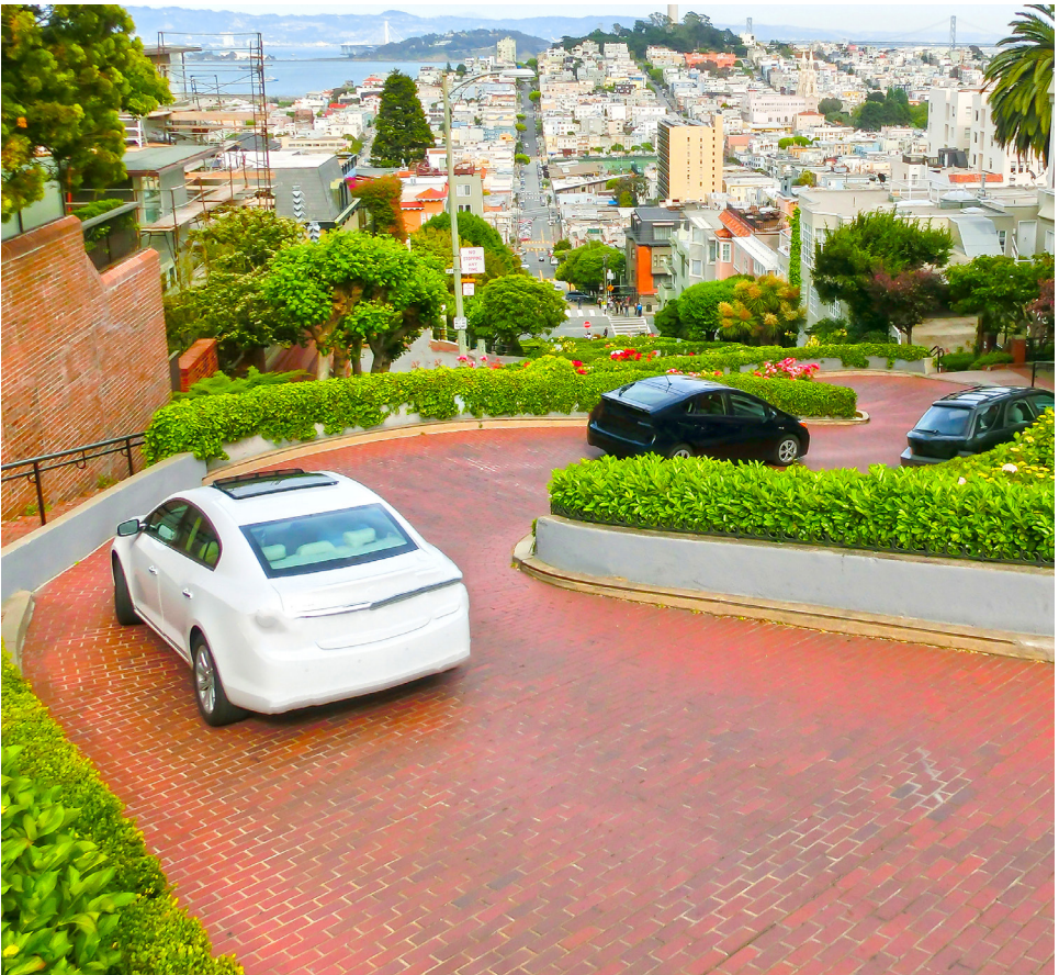
Lombard Street – San Francisco, CA – Installation of thick bed quarry pavers on roadway utilizing the LATICRETE Thick Bed System.
