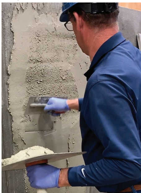
Figure 7.15 – Latex fortified render is being applied to wall surface. Notice the lath strips that are set into the mortar. The lath strips are leveled and plumbed to establish the correct wall render depth. Once the render achieves a sufficient cure, the lath strips are carefully removed and the cavities are filled with mortar.
