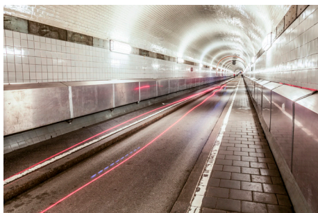
Figure 5.16 – Tiled pre-cast vertical panels in Old Elbe Tunnel, Hamburg, Germany
