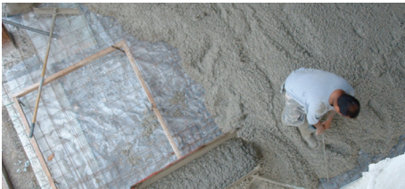
Figure 2.15 – Placement of vapor retarder over blatter layer / directly under the concrete pour. Notice the mechanic pulling the reinforcement wire to the middle of the concrete pour.
